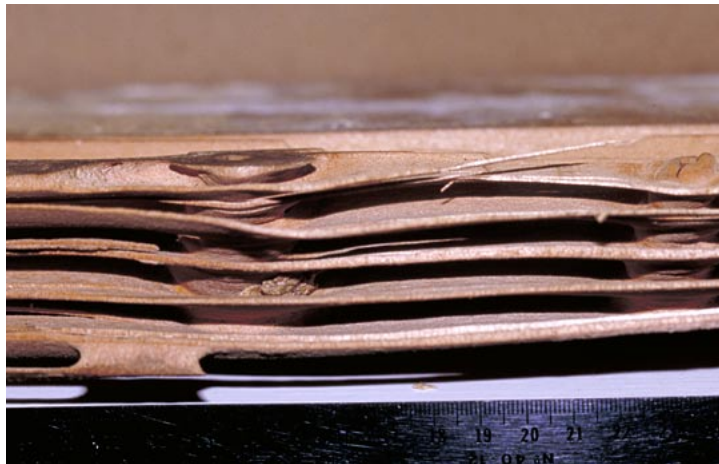
Figure 3. Side view of subfloor plank excavated by carpenter ants.
